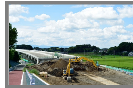
Renovation Demand for Social Infrastructure (Highways) in 2020 (for some 90% of 3 Tokyo metropolitan beltways)
